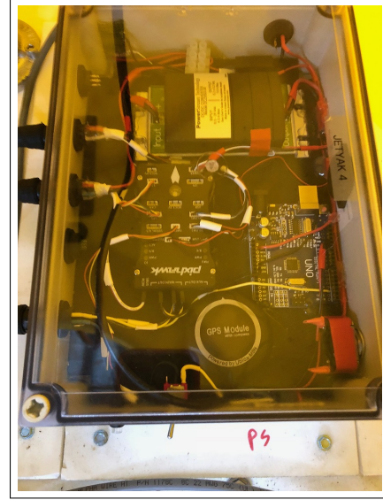
Fig. 5. Electronics box of the ASV, which contains controllers and sensors, including GPS and Arduino. Each of the components can be a source of noise.
